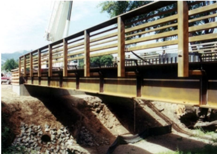
Rebar is added and concrete deck is poured and finished, sidewalk will be added in second pour
