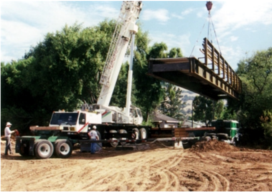
Large sections of bridge are delivered fully prefabricated to subdivision in Novato, CA
